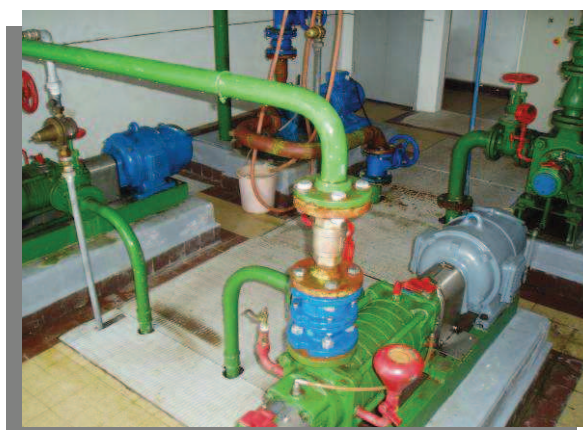
Station de pompage – Photo EPTB Saône et Doubs
